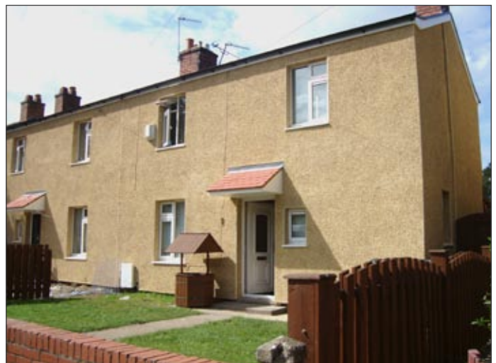
Social Housing Refurbishment Project: Heavy Duty NSC3 EWI System with Dash Aggregate finish
